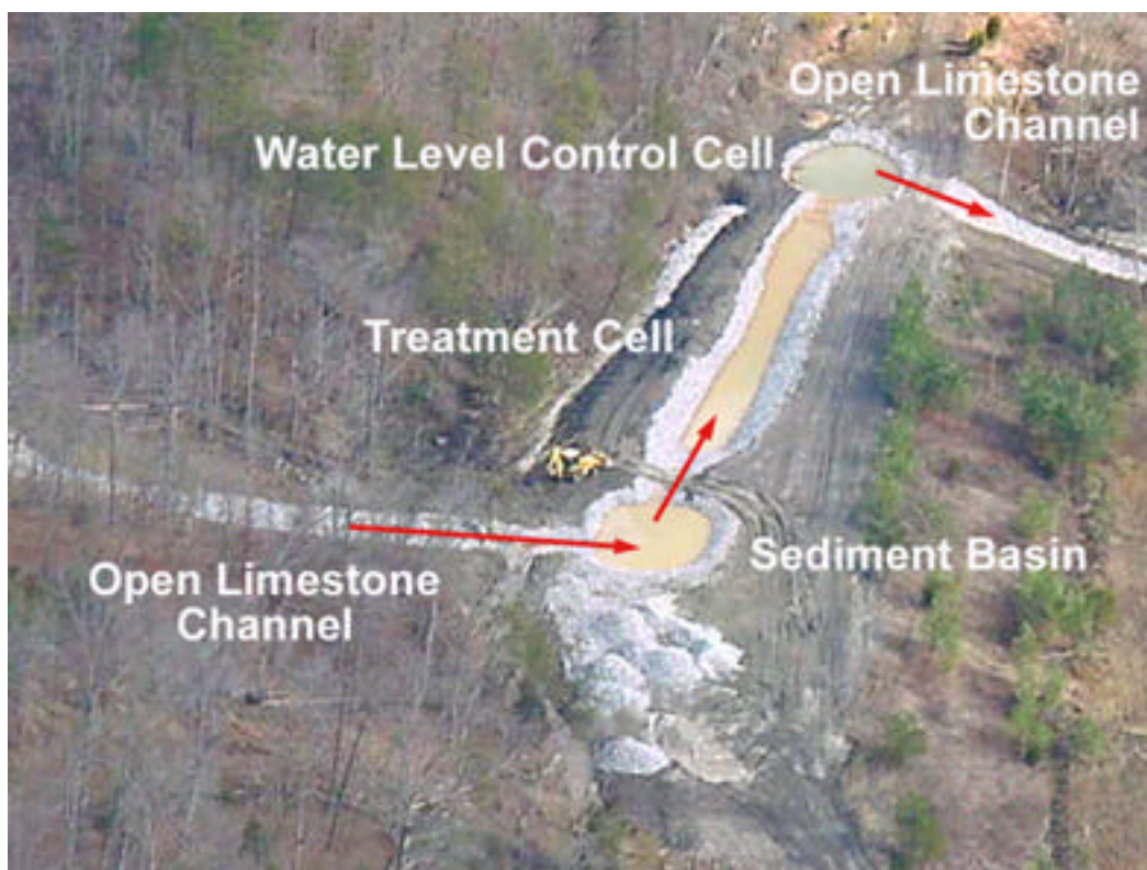
Figure 5. Paint Cliff Vertical Flow System components.
